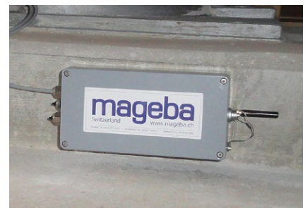
Data acquisition unit of a SHM system
