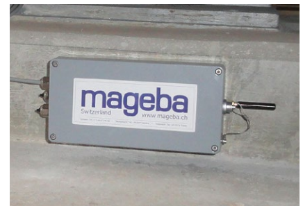
Data acquisition unit of a monitoring system
